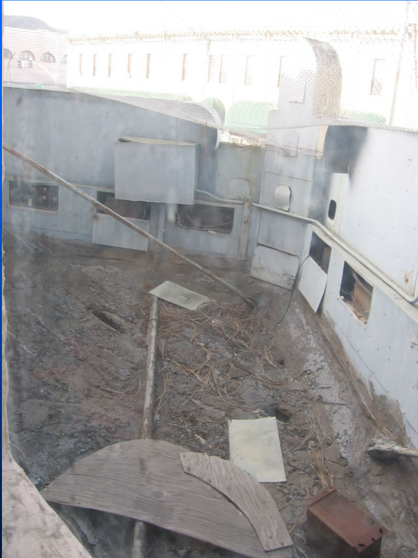
Deterioration & Rot in Top of Marquee
