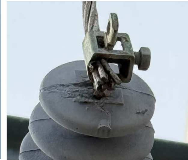
Figure 10: Potential transformer damage
