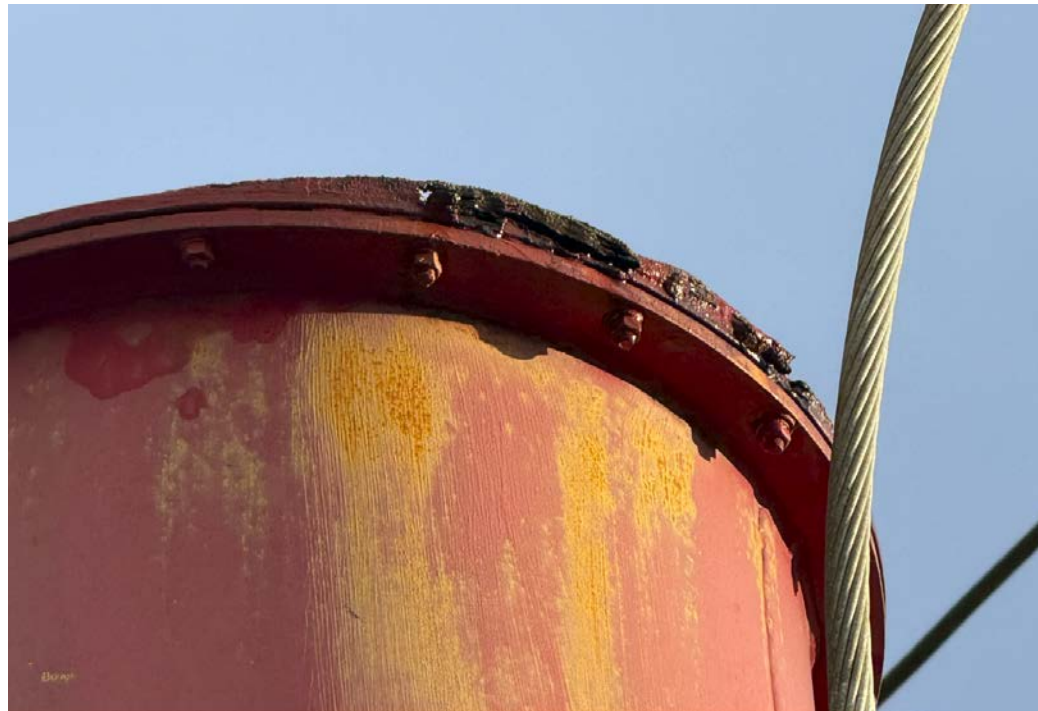
Figures 5 and 6: Lompoc Receiving Station VT/CT lids are deteriorating with rust and swelling risk of water penetration
