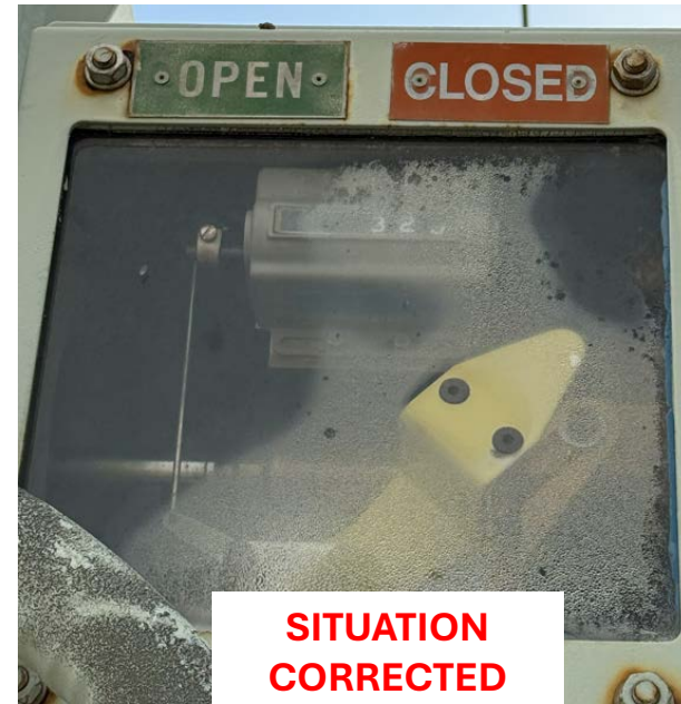
Figure 8: SF6 Circuit Breaker window with moisture
