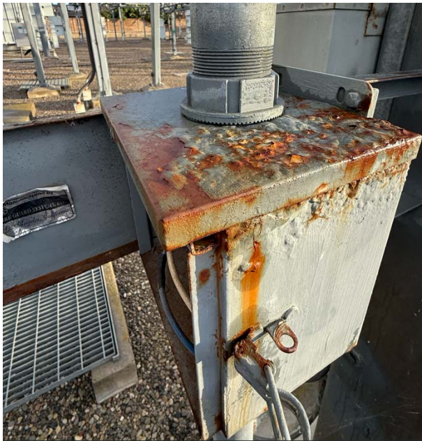
Figure 7: VT/CT junction box with rust
