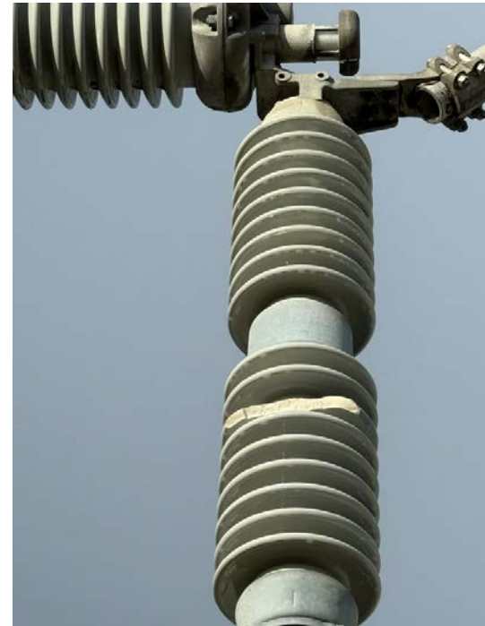
Figure 9: SF6 Circuit Switcher with broken skirt
